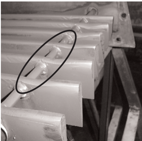
Figure 6 - No protective cladding on the flow element
